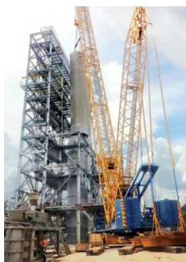
Emerald Kalama upgraded its plant in Rotterdam, the Netherlands, in 2017.
